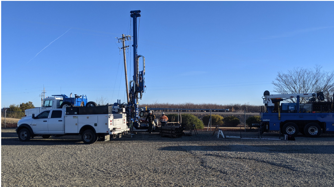
Photo 4: View of Dunnigan Pipeline alignment looking east from Richie Bros. Auction Yard (Alternatives 1, 2, and 3)
