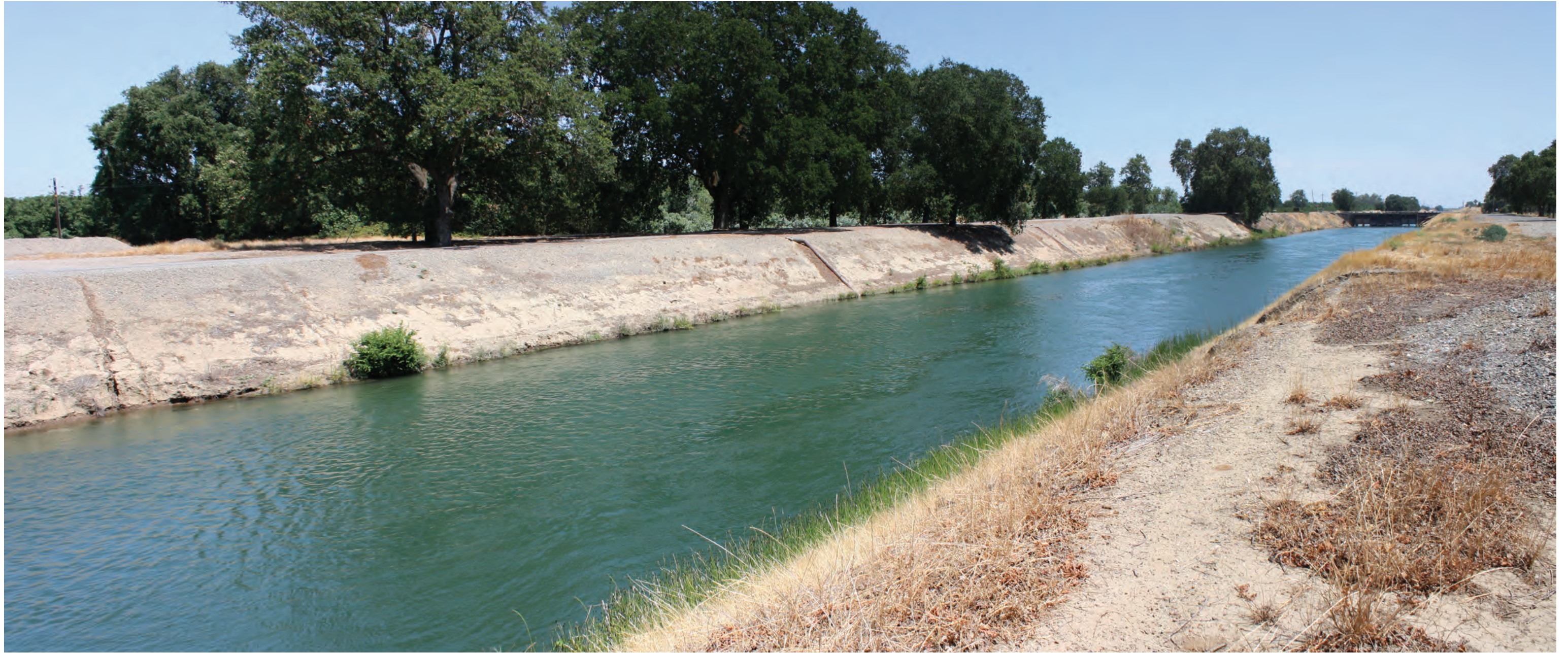
Photo 23: Looking east and southeast toward the proposed GCID Canal Headgate Structure and Canal Lining location from the west side of the GCID Canal.
