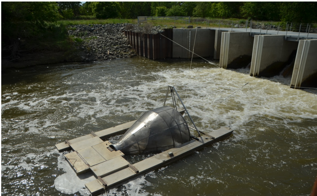
Figure 6. Installation of the rotary screw trap at Weir 2 in the Sutter Bypass.
